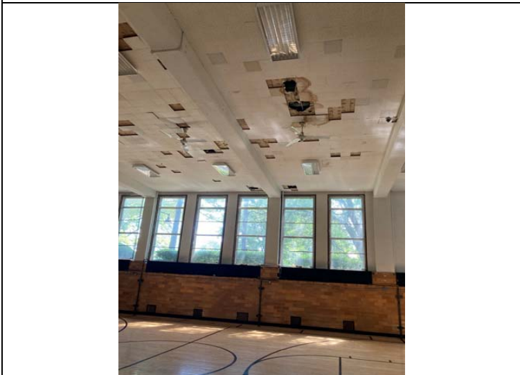
Damaged Ceiling Tiles in the Gymnasium
