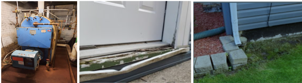
Assessments will address a variety of climate-related features, ranging from boilers in multi-family buildings, to door and window sealing to prevent air leakage, to location of downspouts that may inadvertently cause basement seepage.
