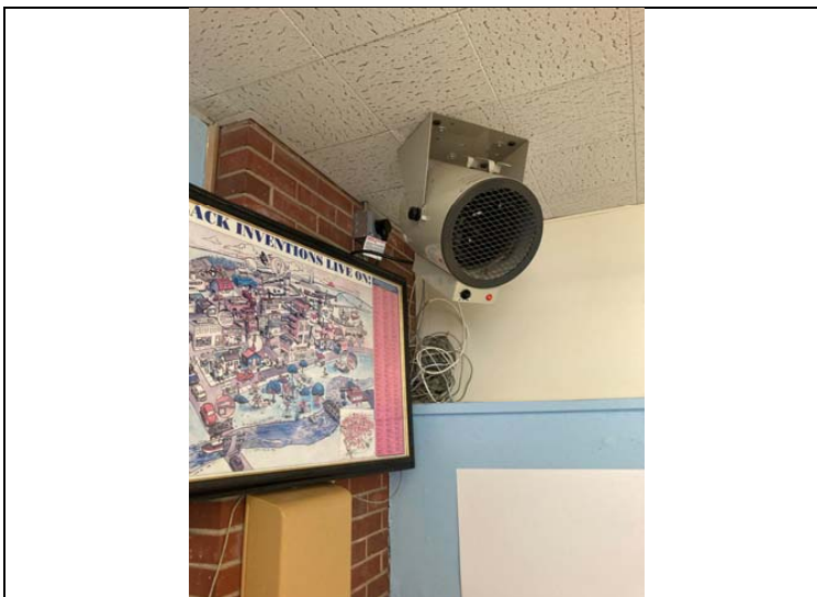
Ceiling Mounted Electrical Heater
