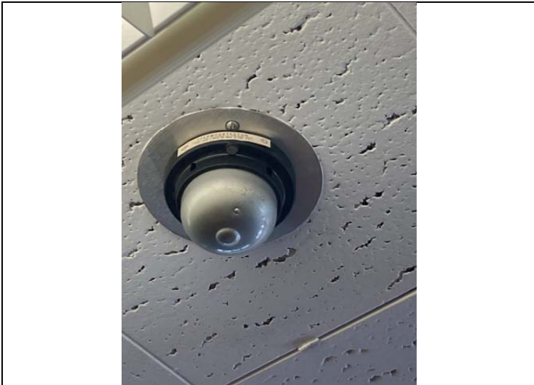
Fire Alarm in Room
